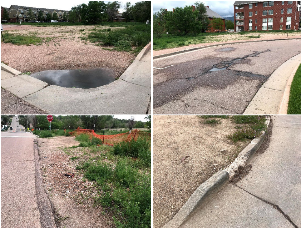
Figure 9. Deteriorated Pavement and Curbs and Missing Sidewalks
