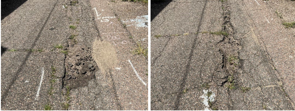
Figure 4. Poor Provision of Street Improvements for Vehicles
