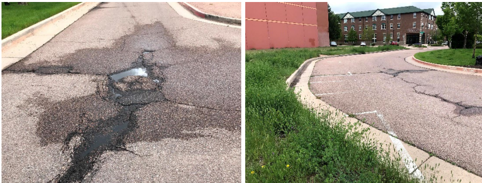
Figure 2. Poor Provision of Street Improvements
